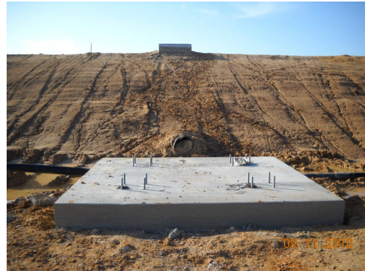
MSI, complete decant pads, PDP 3
