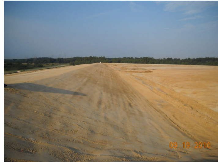
MSI, interior slope protective cover, SE PDP 3
